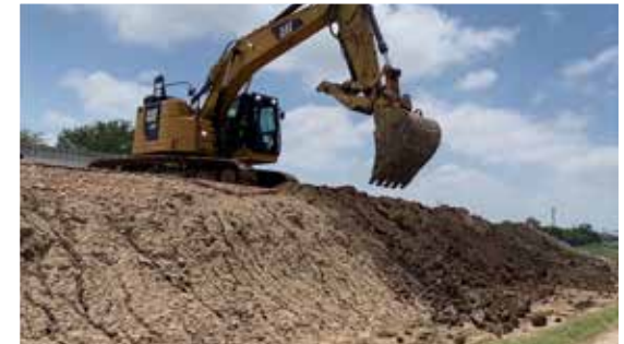
Structural actions such as levees
